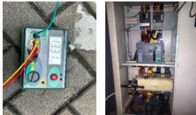
Figure 5. a. Initial grounding-resistance measurement result. b. Distribution-panel condition before grounding optimization
