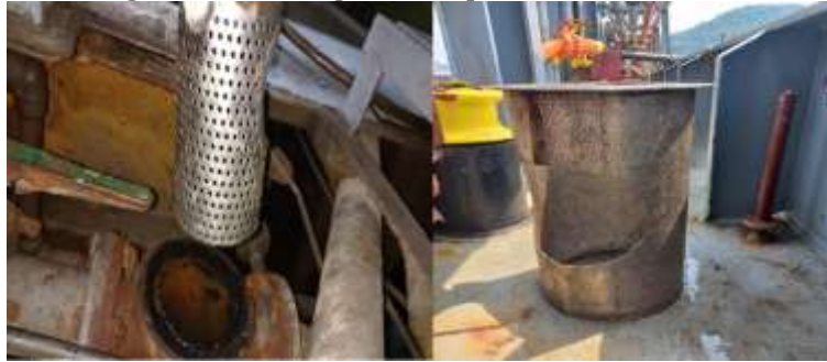
Figure 7 Strainer sea chest pump strainer sea water CAT 18 diesel engine Source: Research Document (2024)
