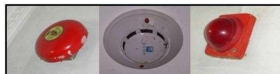
Gambar 4.19 Fire alarm sistem
