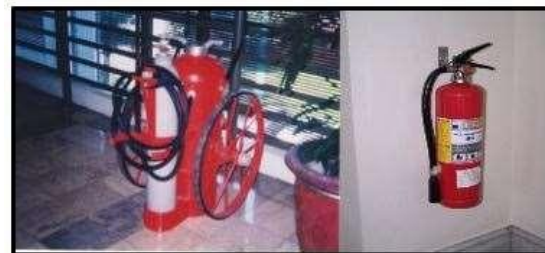
Gambar 4.22 APAR (Alat Pemadam Api Ringan) Sumber : Azizah, Fire Protection, hand Out, 2011
